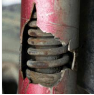
Image: A close-up of a severely rusted and damaged old strut, indicating the need for replacement due to corrosion and structural failure.
