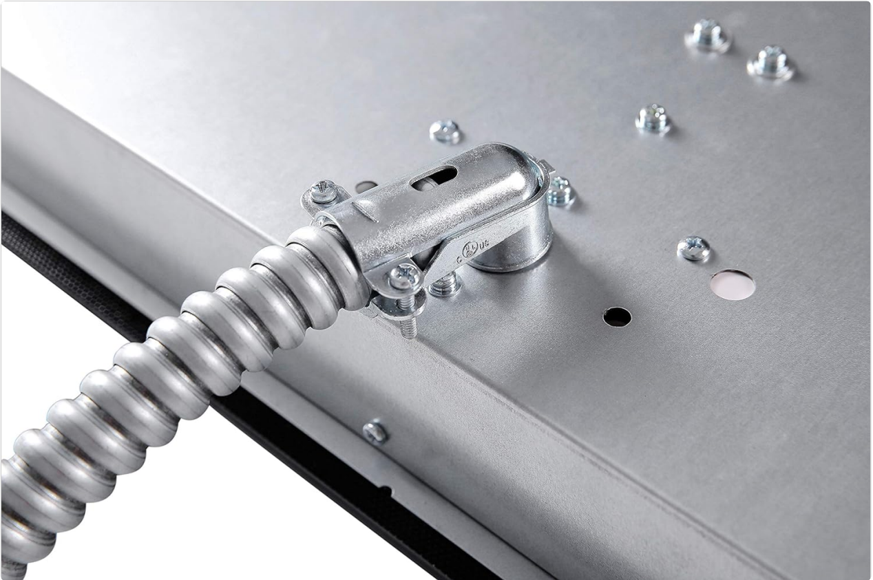
Figure 3.2: Electrical Connection. This image shows the robust electrical conduit provided for hardwiring the cooktop, emphasizing the importance of secure and compliant electrical connections.
