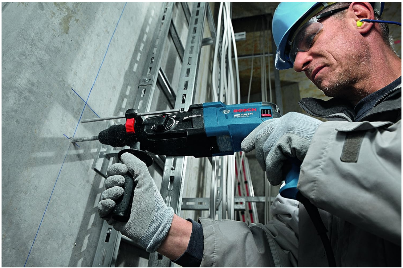
Figure 4.2: An operator demonstrating proper two-handed grip while drilling into a concrete surface.
