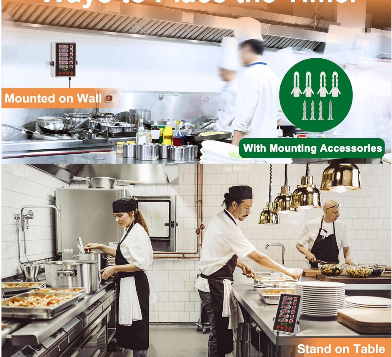
Figure 5: The timer can be mounted on a wall or placed on a table using its adjustable stand, offering versatile installation options.
