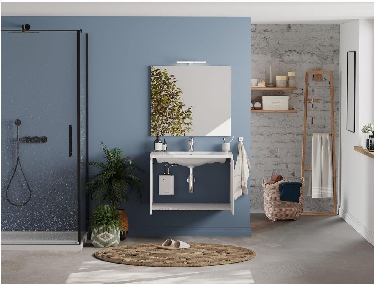
Figure 2: Thermoflow Elex 3.5 kW Instantaneous Water Heater installed under a sink in a bathroom setting.
