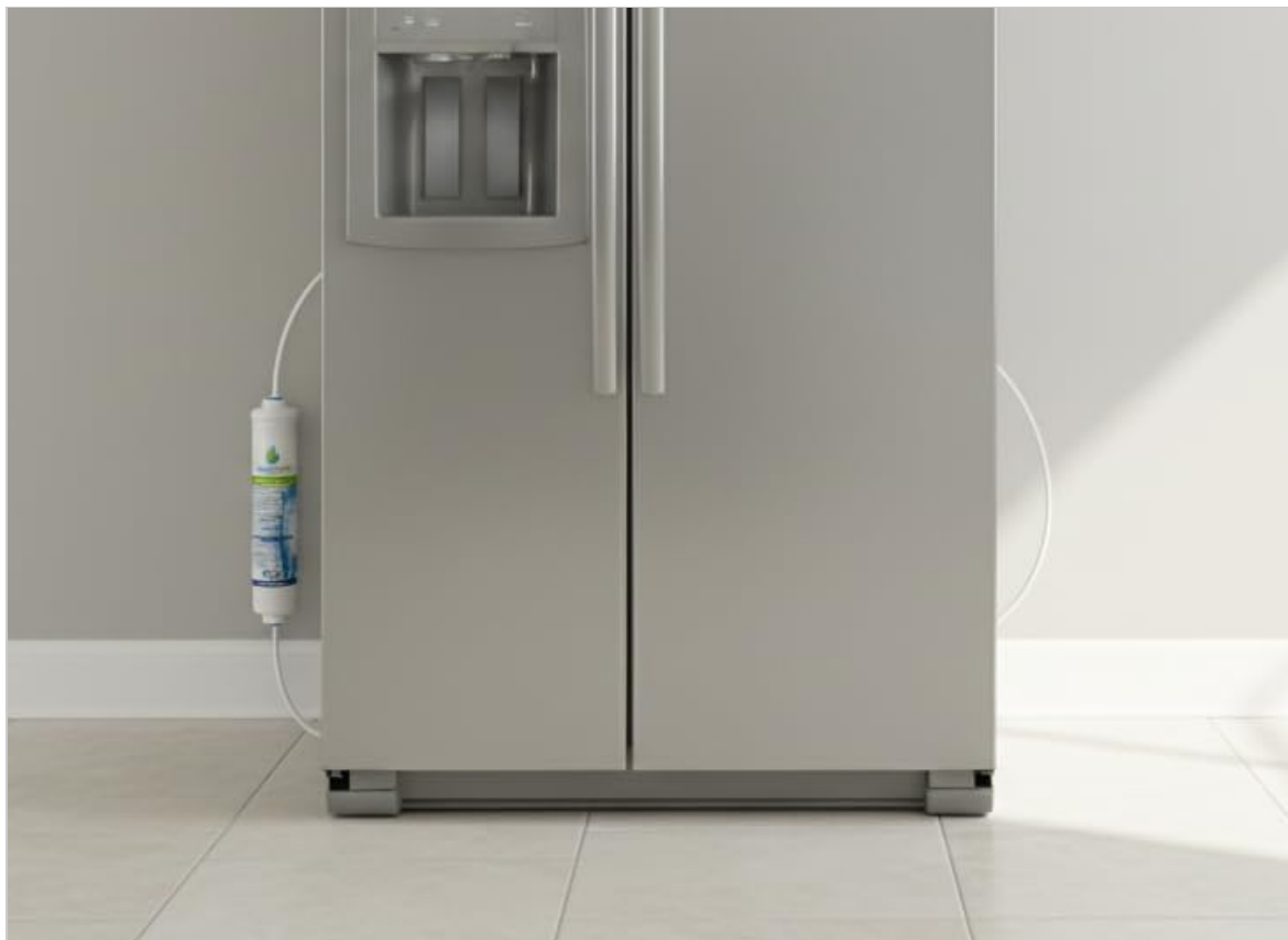
Image: AquaHouse AH-UIF filter installed next to a refrigerator, showing its inline connection to the water supply.
