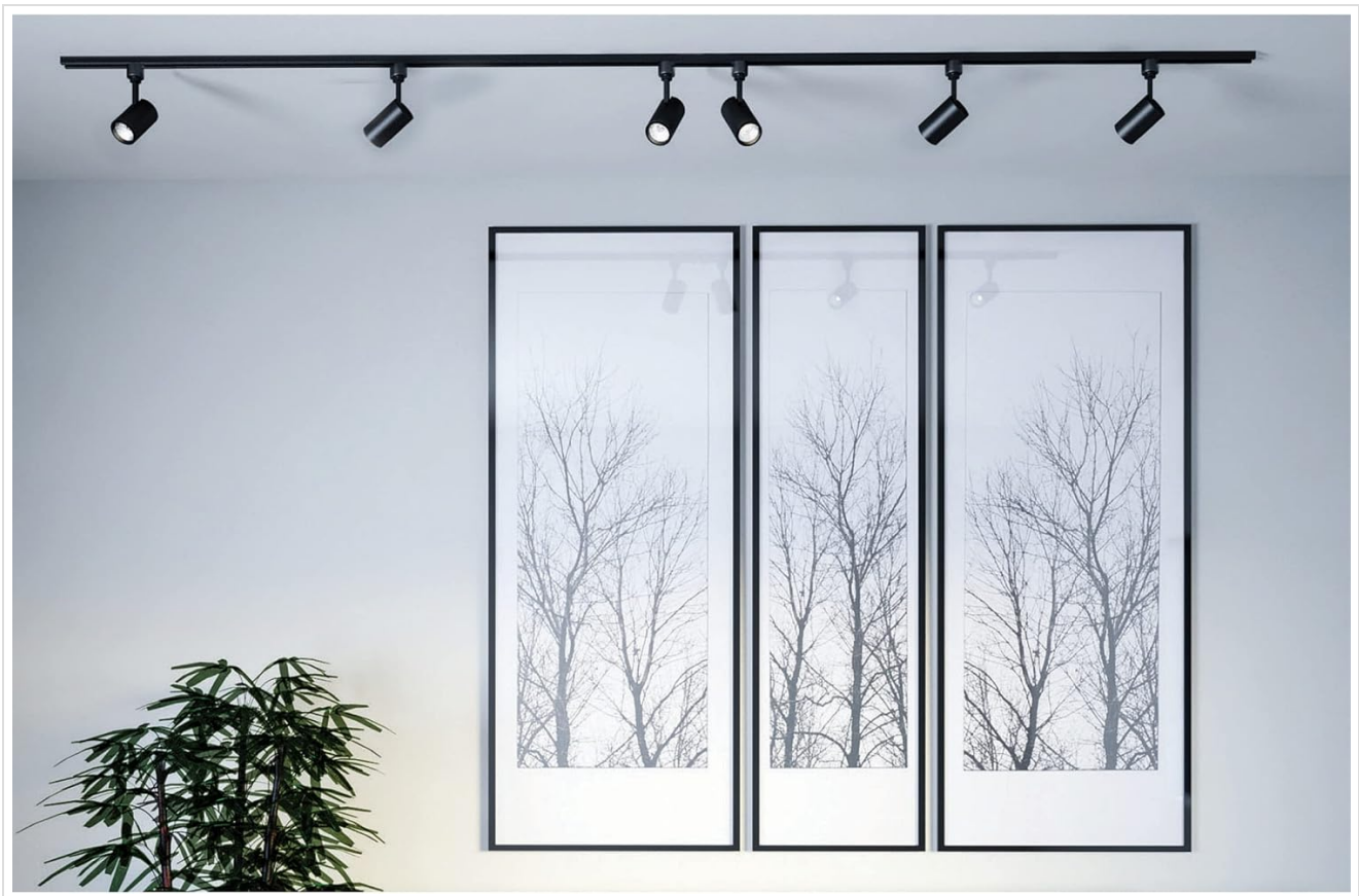
Figure 2: Multiple Nuvo Lighting TH404 LED Track Heads installed on a track system, illuminating a wall with framed artwork.
