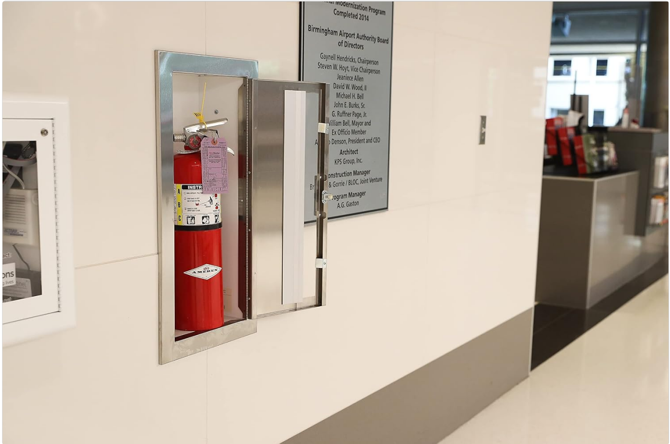
Figure 4: An Amerex fire extinguisher housed within a wall-mounted cabinet, demonstrating a common installation method.
