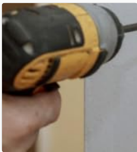
Figure 6: A screwdriver being used to secure the mud ring to an electrical box, utilizing the angled mounting slots.
