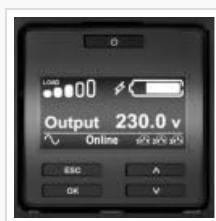
Figure 3.1: A close-up of the UPS LCD display, showing normal operation with an output of 230.0V and the system status as 'Online'.
