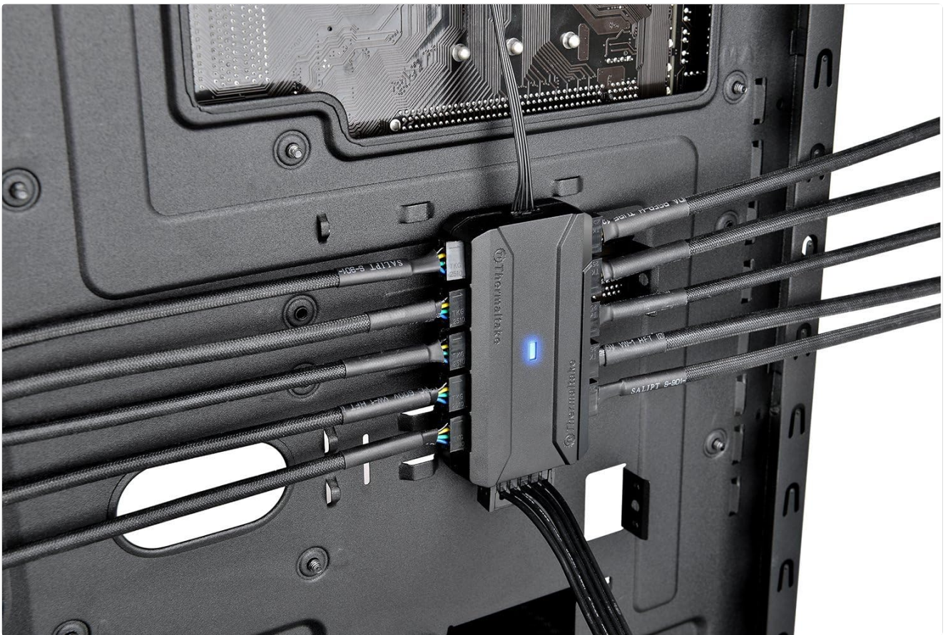
Figure 3: The fan hub neatly installed behind the motherboard tray, demonstrating effective cable management.
