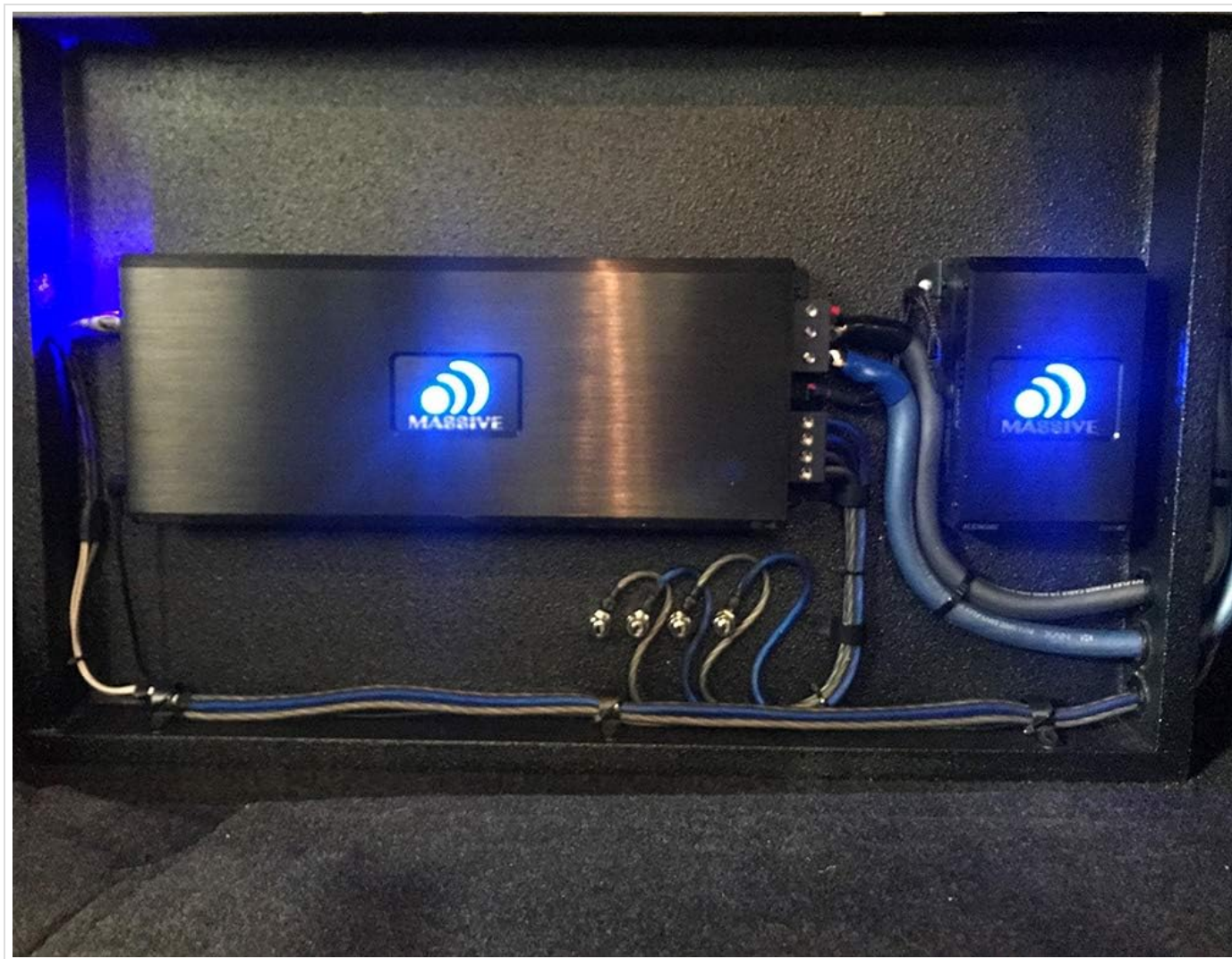
Image 5.1: Example of the amplifier installed in a vehicle trunk, demonstrating a typical mounting scenario with other audio components.
