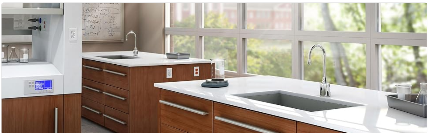
Image: Moen M-Bition faucets installed in a commercial laboratory environment, demonstrating their suitability for professional spaces.
