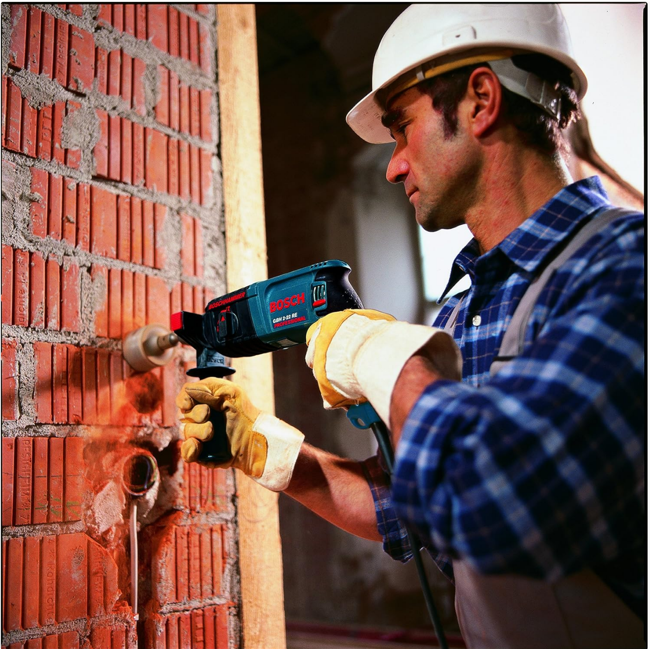
Figure 5.2: Demonstrating the use of the rotary hammer for drilling into a brick wall.
