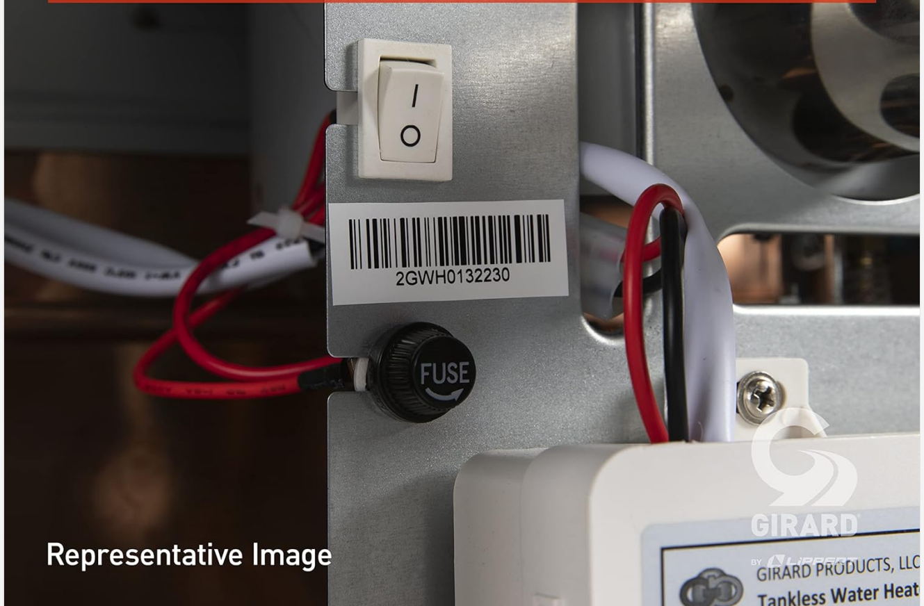
Figure 5: Internal components demonstrating the system's ability to maintain consistent water temperature.
