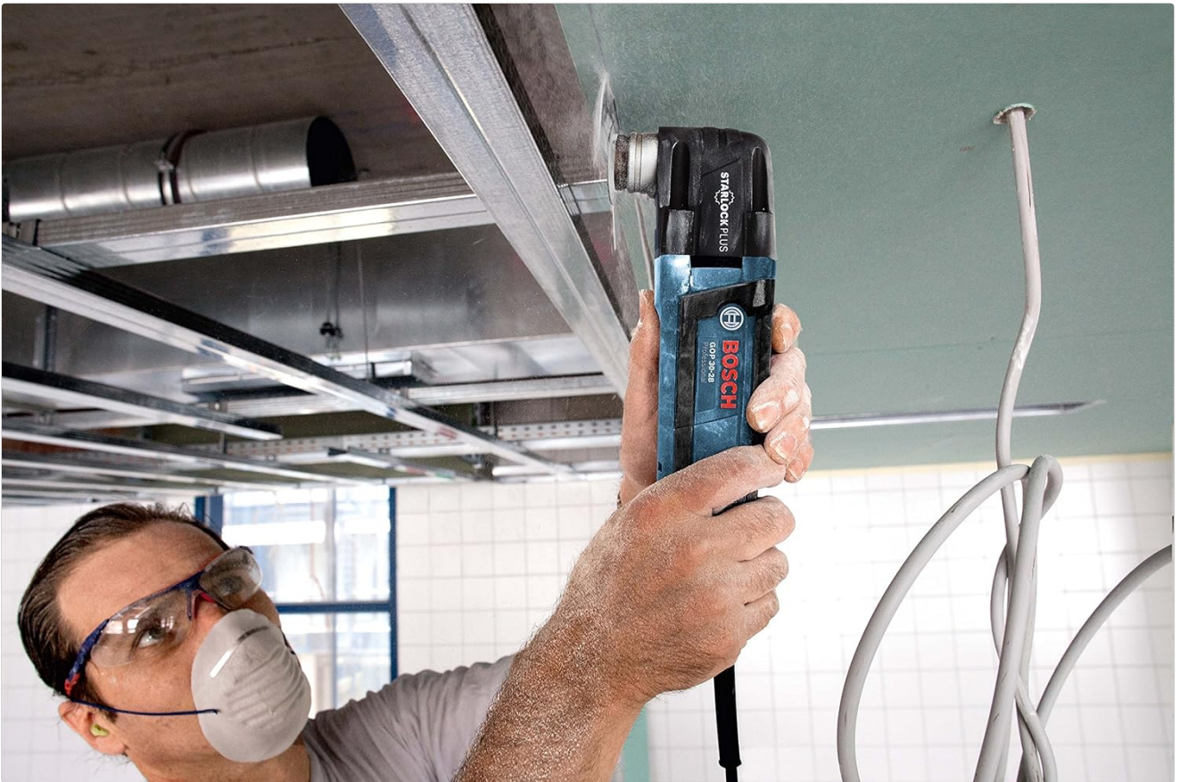
Figure 5.2: An individual utilizing the multi-tool for cutting a ceiling panel, demonstrating overhead application.
