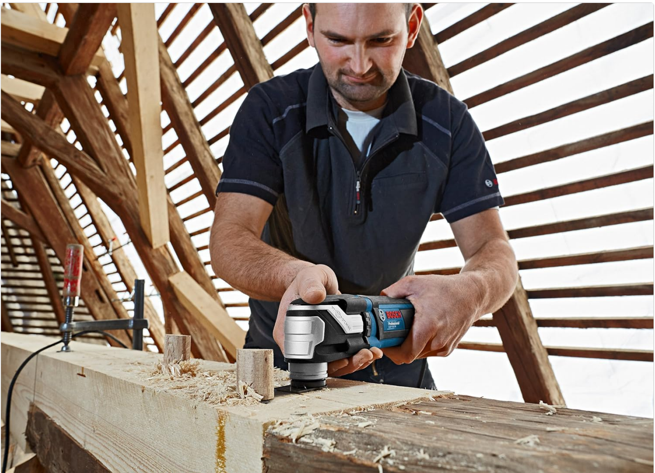
Figure 5.3: A worker performing sanding operations on a wooden beam with the Bosch GOP 30-28 Multi-Tool.
