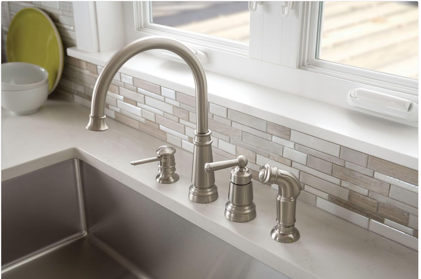
Figure 3: The Moen Edison kitchen faucet, side sprayer, and soap dispenser elegantly installed on a kitchen sink, demonstrating its functional integration into a modern kitchen environment.
