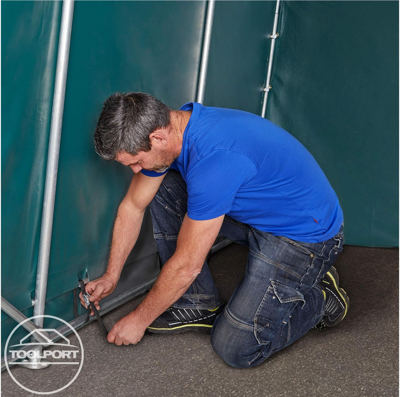
Image 3: Securing the base of the shelter to the ground using provided fasteners.
