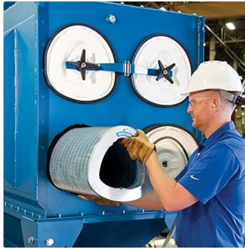
Figure 3.1: A technician performing an installation, emphasizing the importance of proper handling and secure fitting of components.
