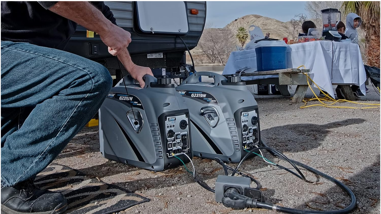
Connecting two Pulsar G2319N generators in parallel to double the power output.
