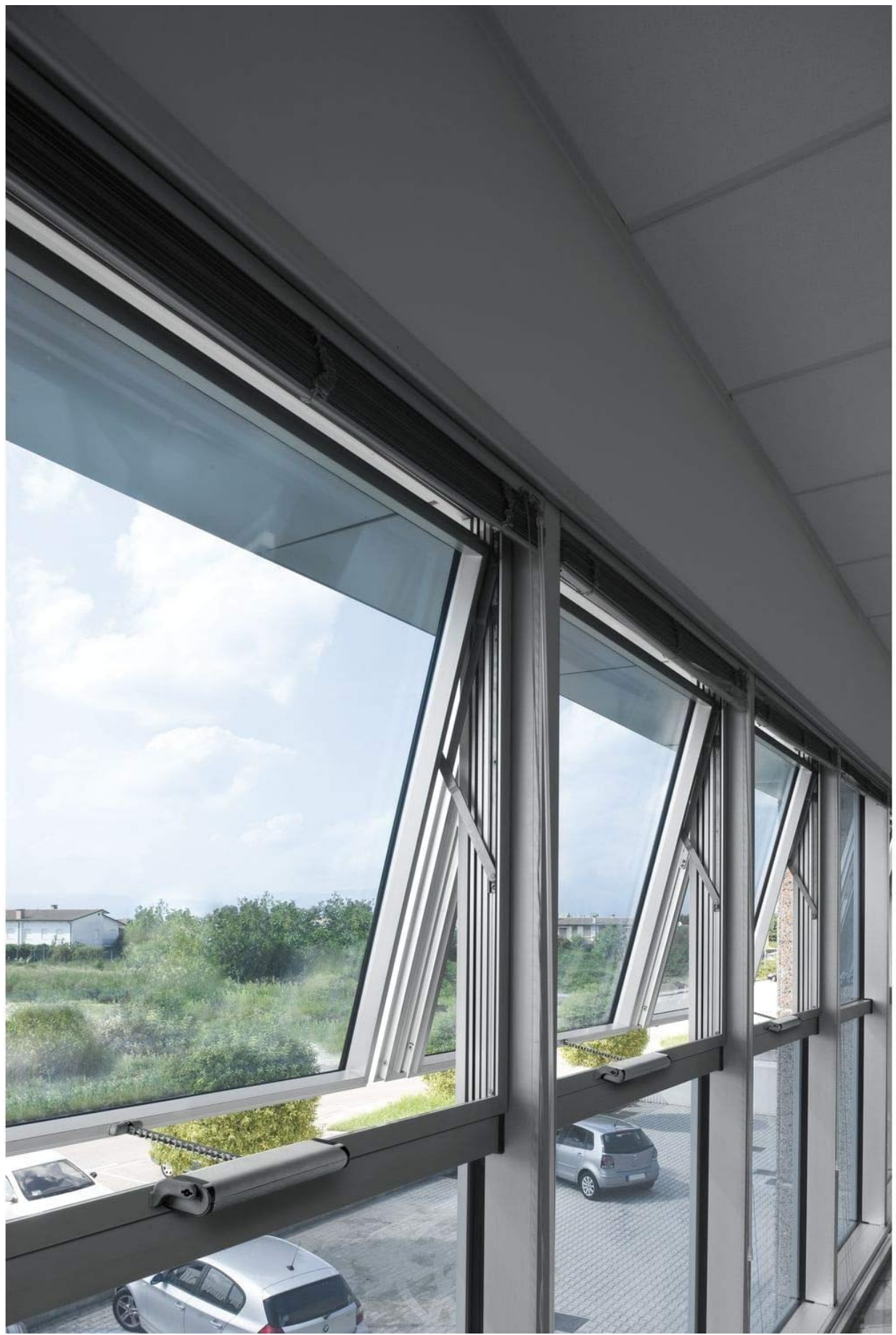
Figure 4: Multiple chain motors operating in parallel on a series of windows.
