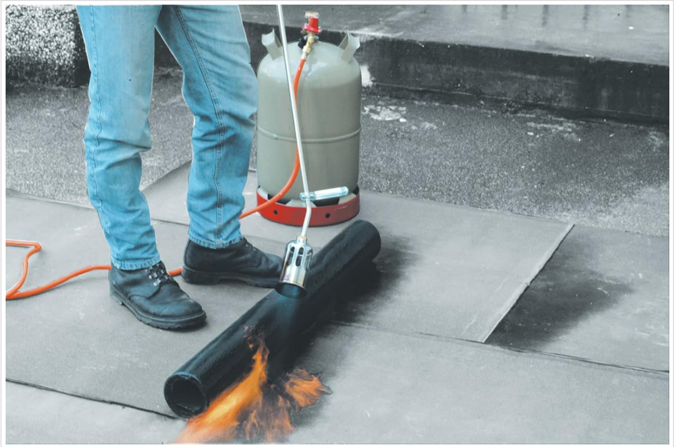
Image 4: An individual using the Rothenberger ROMAXI burner to heat and apply a roofing membrane, showcasing the tool's primary function.
