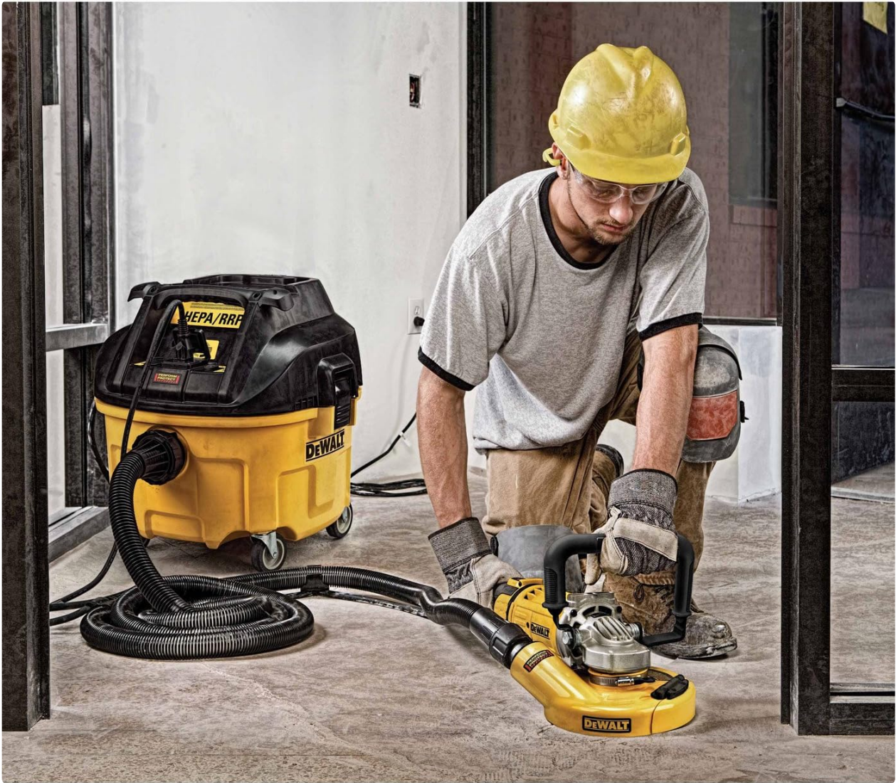
Figure 3: The DEWALT DWV010 Dust Extractor connected to a concrete grinder, demonstrating its application in dust control during construction tasks.
