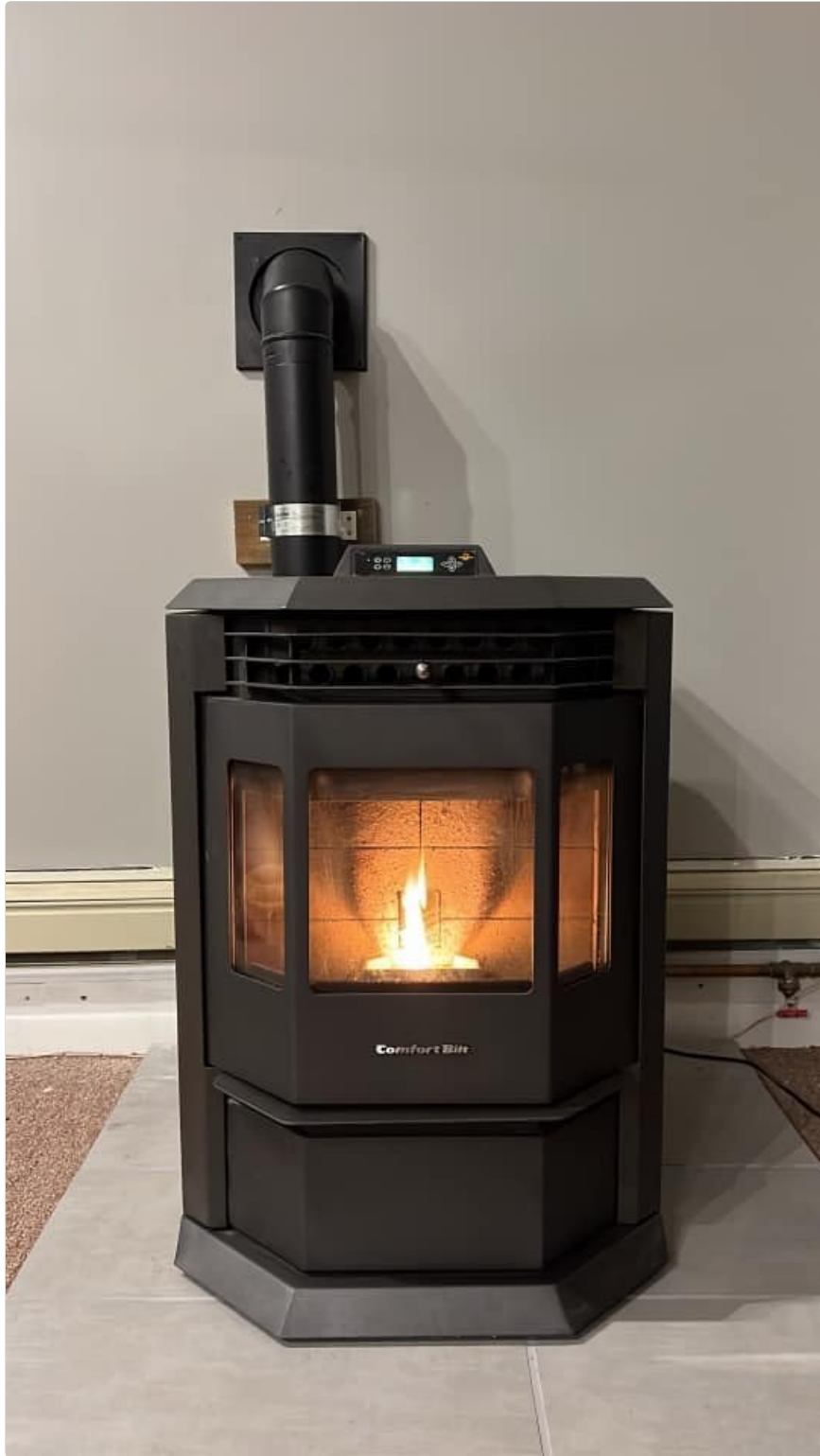
Image: A Comfortbilt HP22 Pellet Stove with a visible flame inside the bay-style viewing window, indicating active operation.
