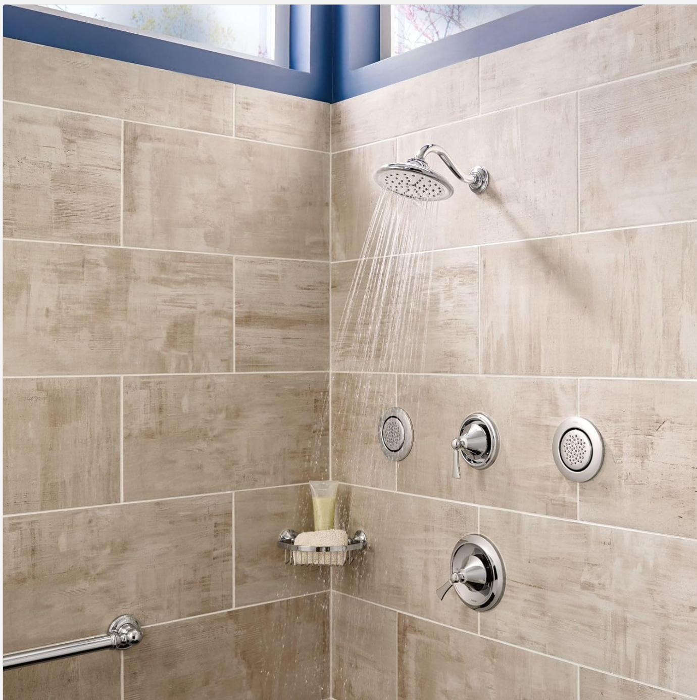
Image 2.1: An example of a Moen Wynford shower system installed, demonstrating the integration of the valve trim with other shower components.
