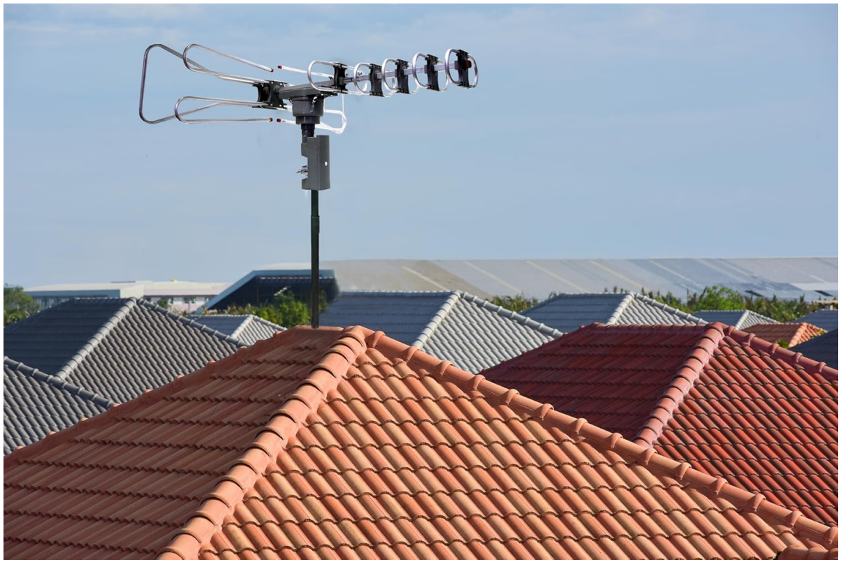
Image: Naxa NAA-350 antenna installed on a rooftop, demonstrating typical outdoor placement for optimal signal reception.
