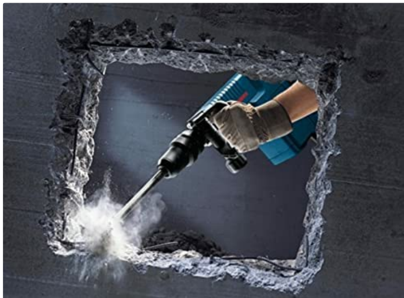
Image: The Bosch GSH 11 E Demolition Hammer in action, effectively breaking through a concrete surface, demonstrating its powerful impact.
