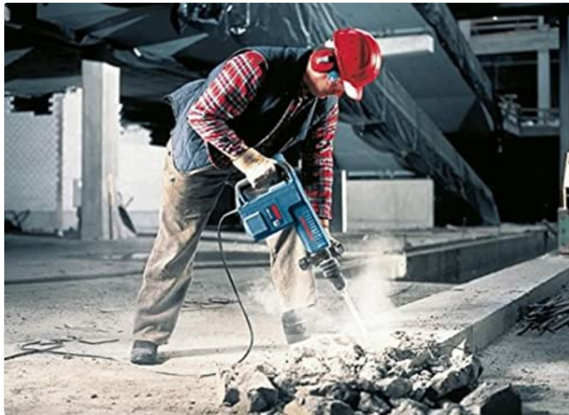
Image: A worker wearing safety gear operates the Bosch GSH 11 E Demolition Hammer to break up rubble on a construction site, highlighting its heavy-duty application.
