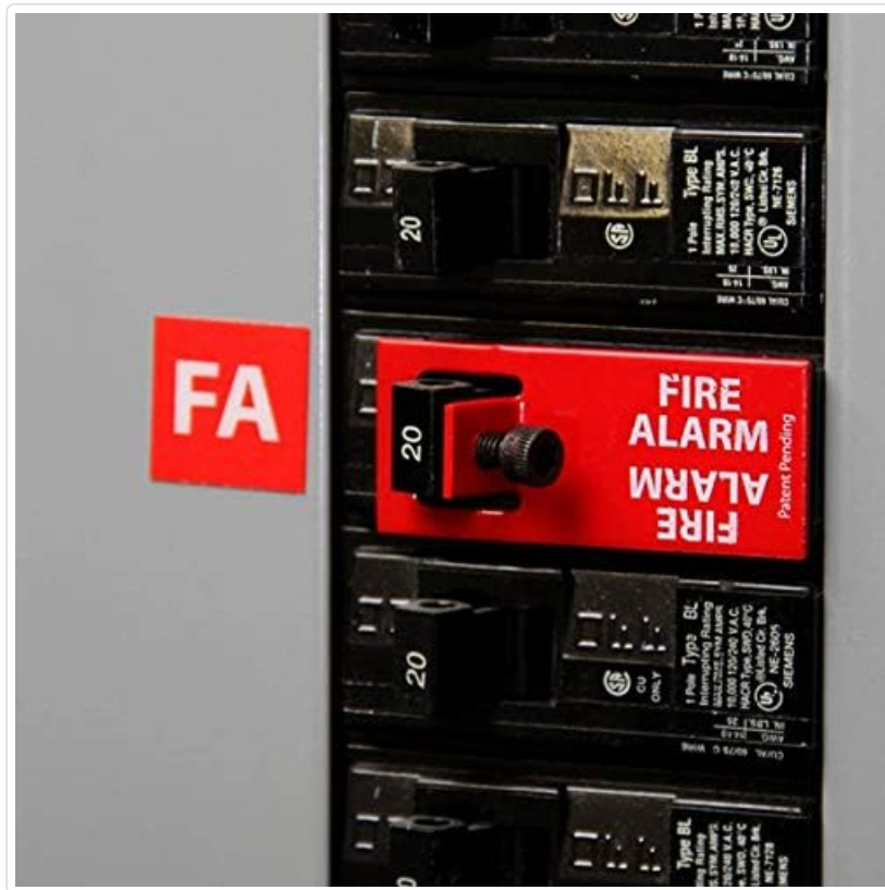
Figure 3: Close-up view of the ELOCK-FA lockout tab and "FA" label correctly installed on a circuit breaker within a panel. This image demonstrates the secure placement of the lockout device and the clear identification of the fire alarm circuit.
