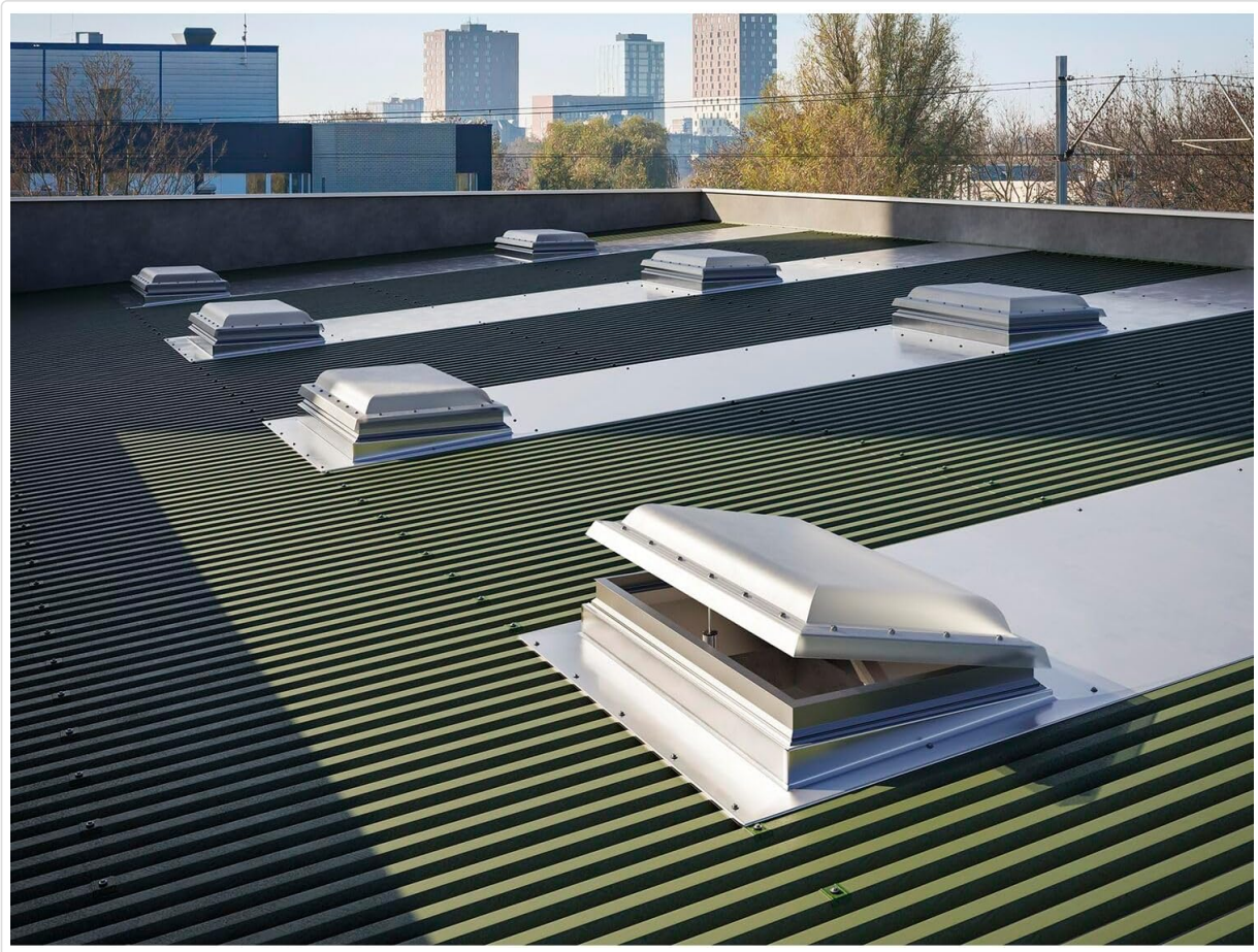
Figure 4: Multiple roof windows equipped with COMUNELLO actuators for automated ventilation.
