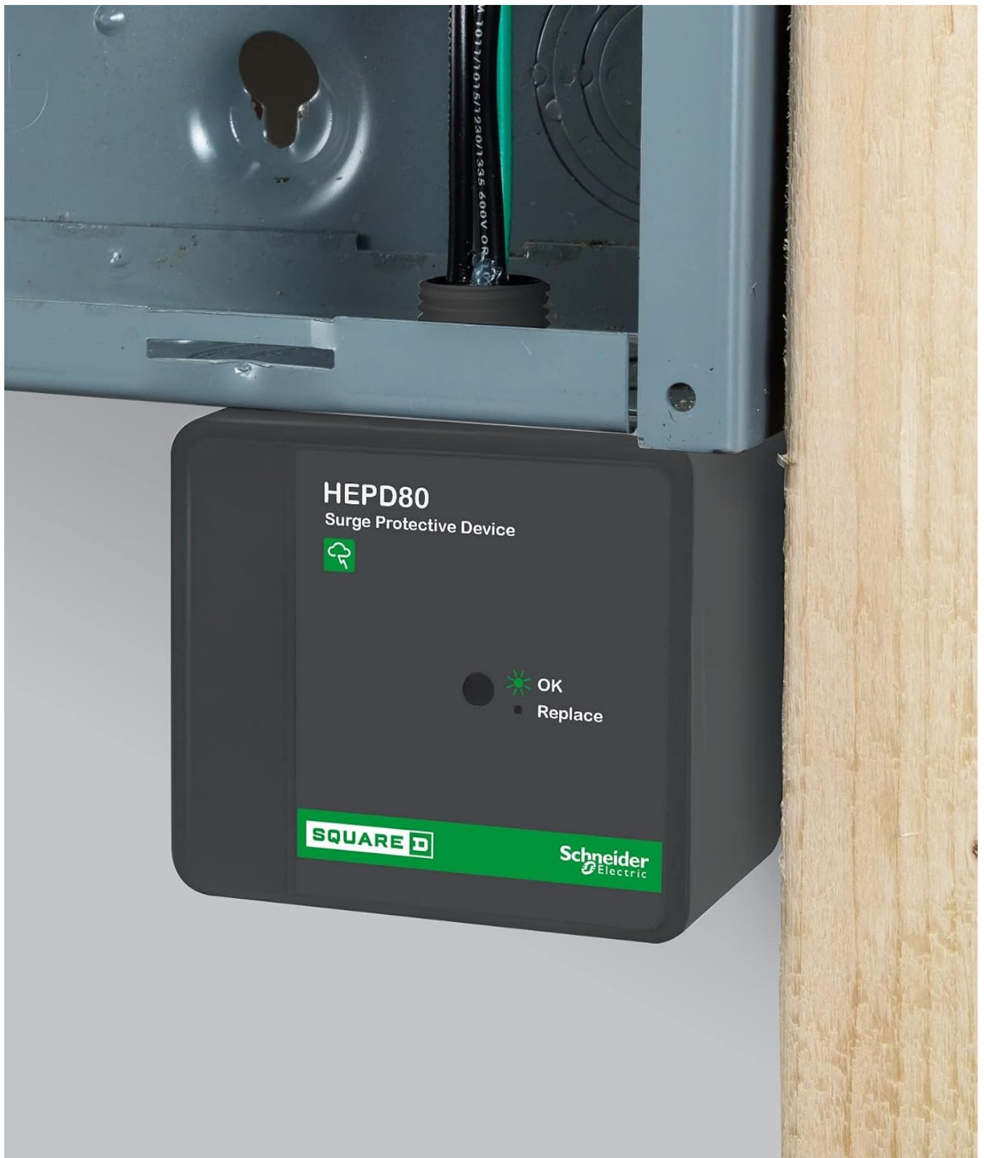
Image 2: The HEPD80 device mounted to an electrical panel, showing its connection point.
