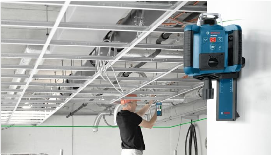
Figure 3: The Bosch LR1G receiver being used in conjunction with a rotary laser to establish a level line on a construction site.
