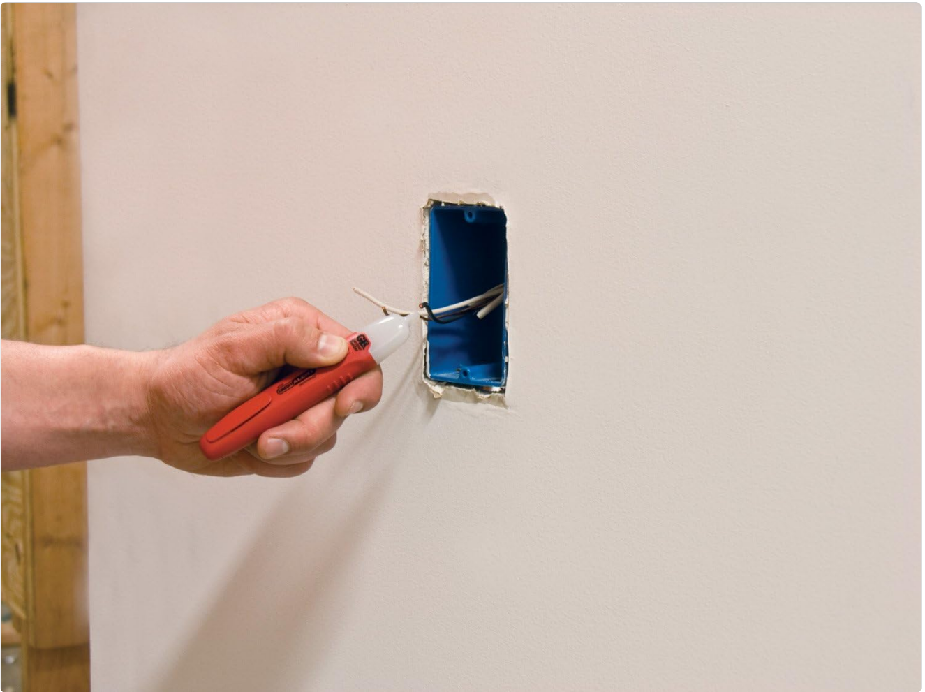
Figure 3: Using the GVD-3504 to test wires for voltage.
