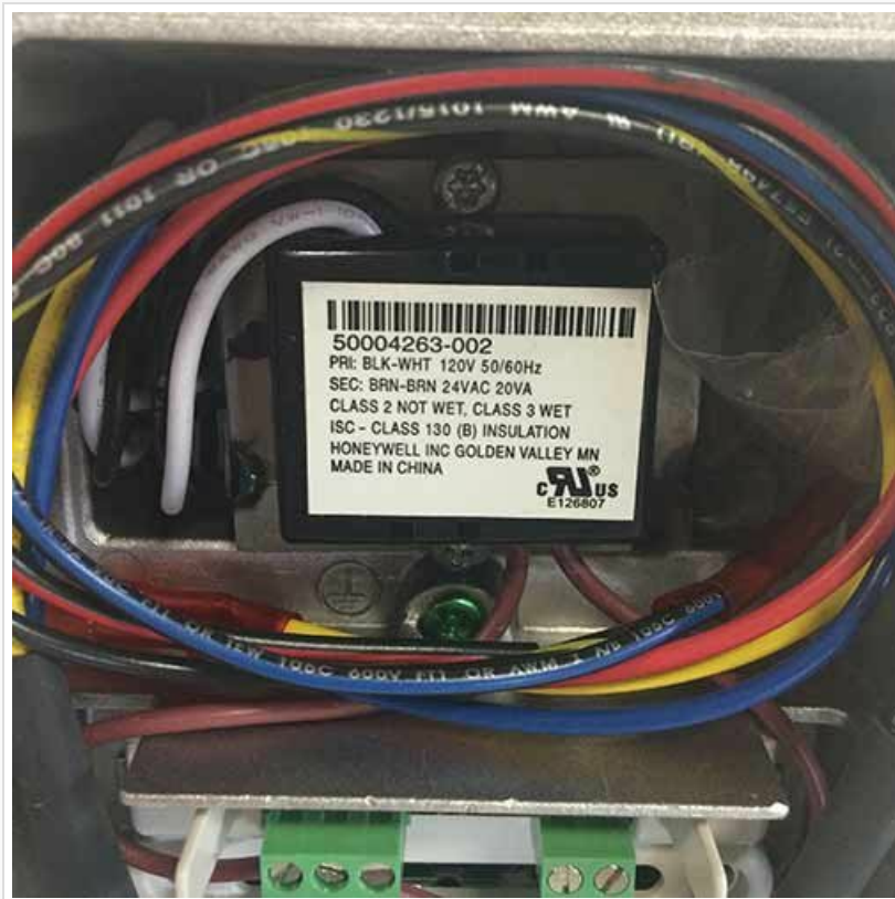
Figure 5: Close-up of the internal label detailing electrical specifications and manufacturer information.
