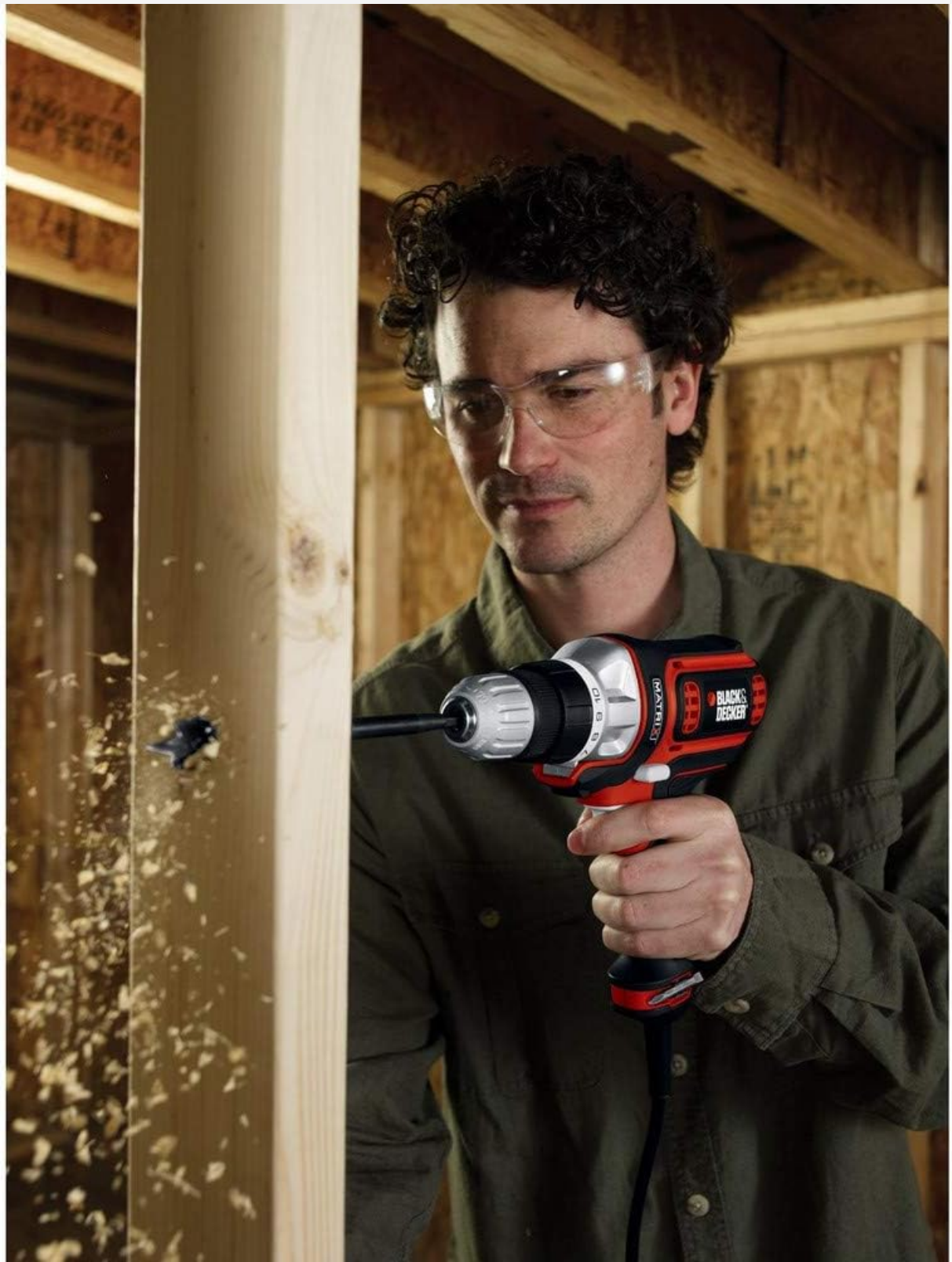
Image 5.3: A user drilling a larger diameter hole into a wooden beam, illustrating the drill's capability for more demanding tasks.
