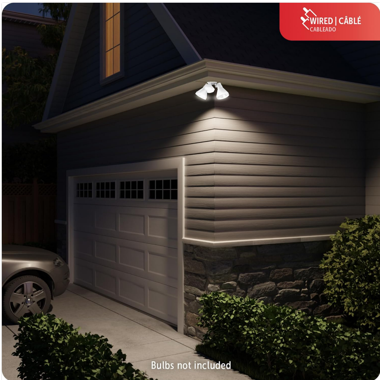
Figure 4: Example of the security light installed above a garage.
