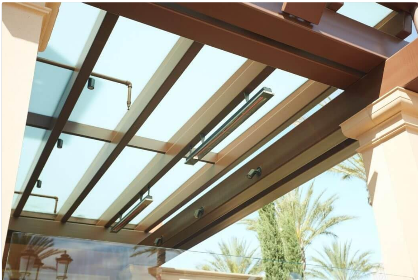
Figure 3: Multiple Infratech heaters installed under a glass roof structure, illustrating overhead mounting for outdoor dining areas.
