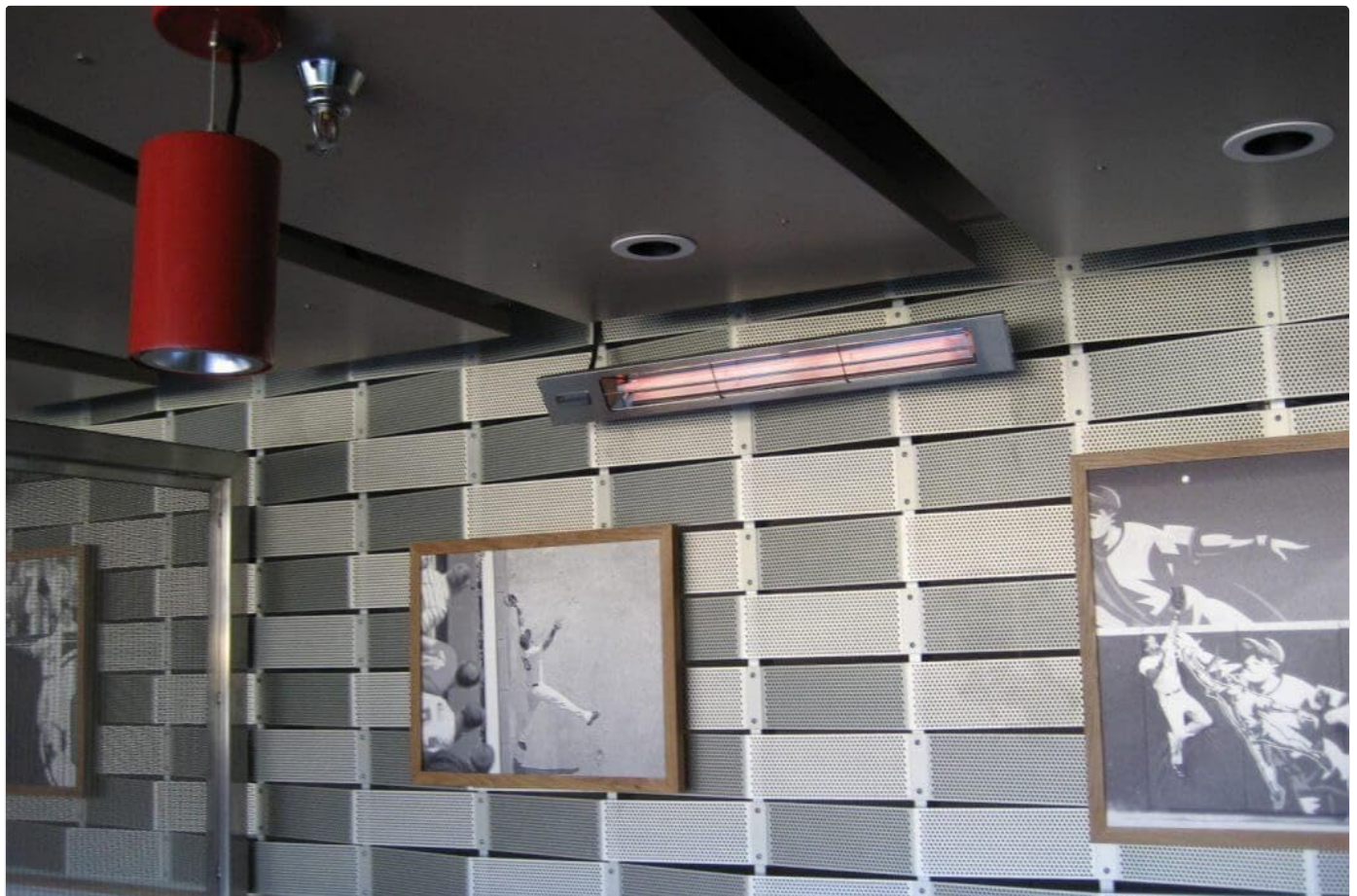
Figure 2: An Infratech heater mounted on a wall, demonstrating a common installation scenario in an indoor/outdoor setting.
