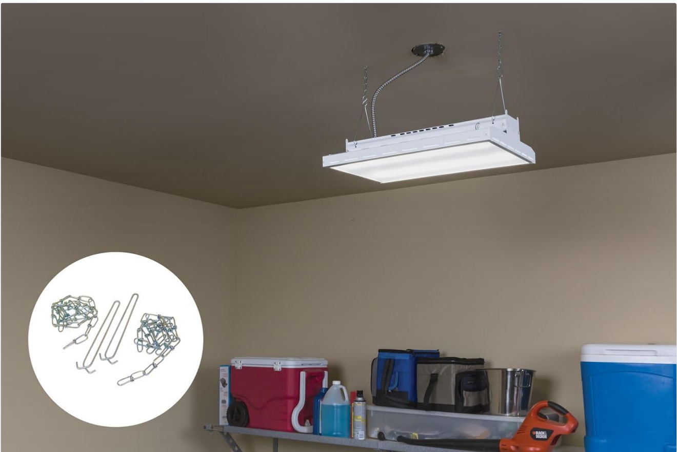
Image 5.2: An example of a light fixture successfully installed and suspended in a garage environment using the chain kit.
