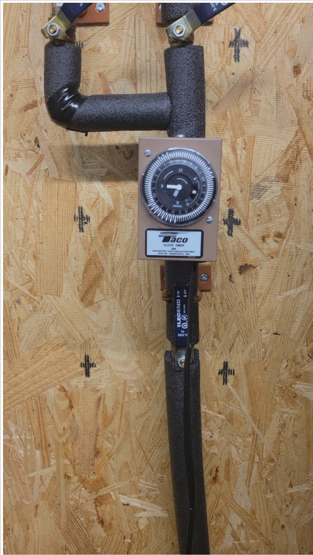
Figure 2: Taco T265-1 Analog Timer installed on a domestic hot water recirculation system. The timer is mounted on a wall, connected to insulated piping leading to a water heater. This illustrates a typical installation scenario.
