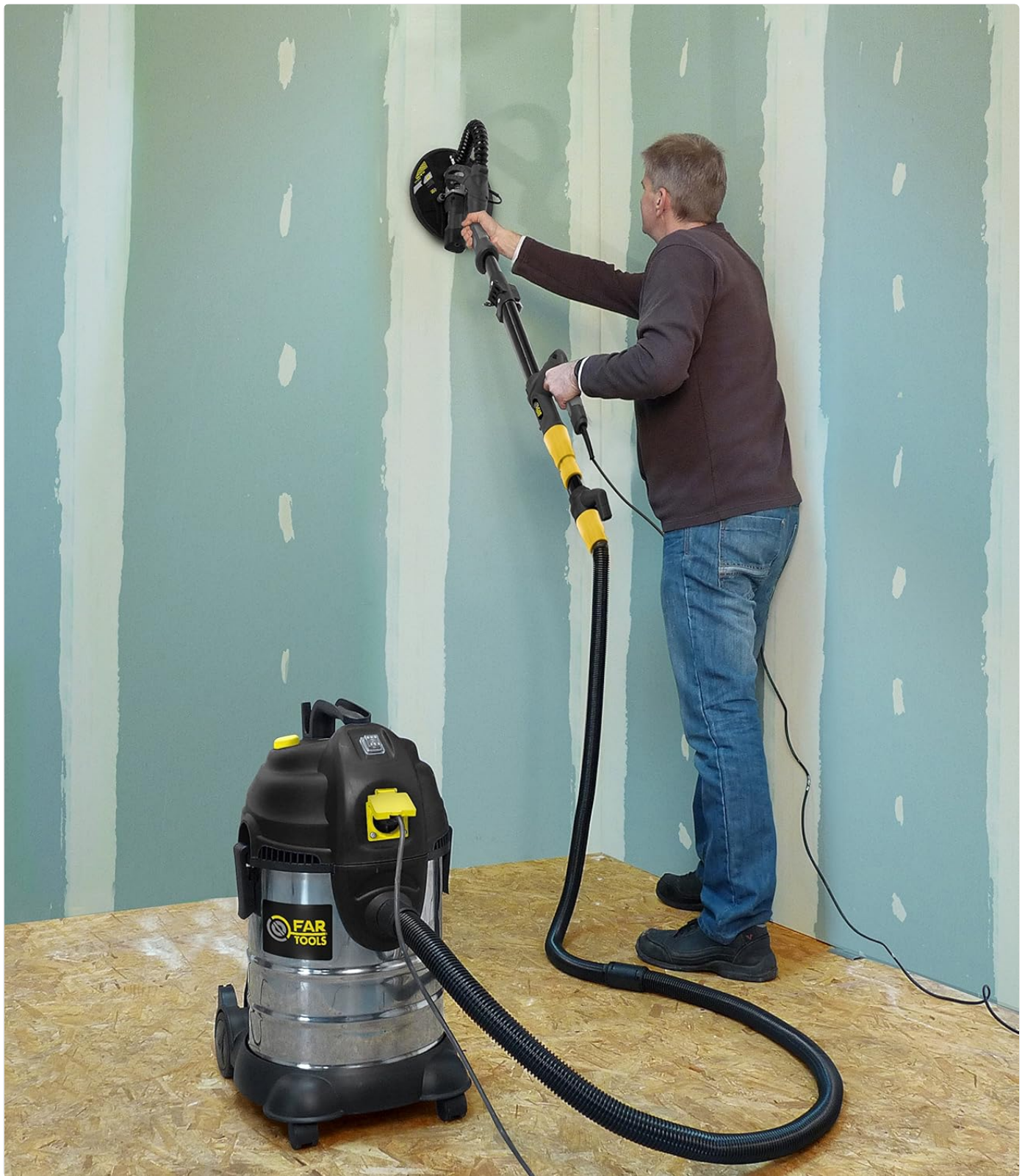
Image 4.1: An operator using the Far tools DWS 710E sander on a wall, with a vacuum cleaner connected for dust collection.
