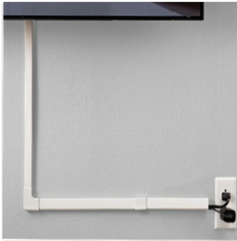
Image: An example of an installed raceway system with cables neatly concealed.
