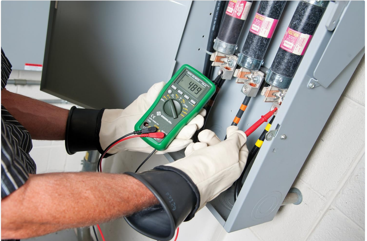
Figure 4: Measuring current in an electrical panel with the DM-45.
