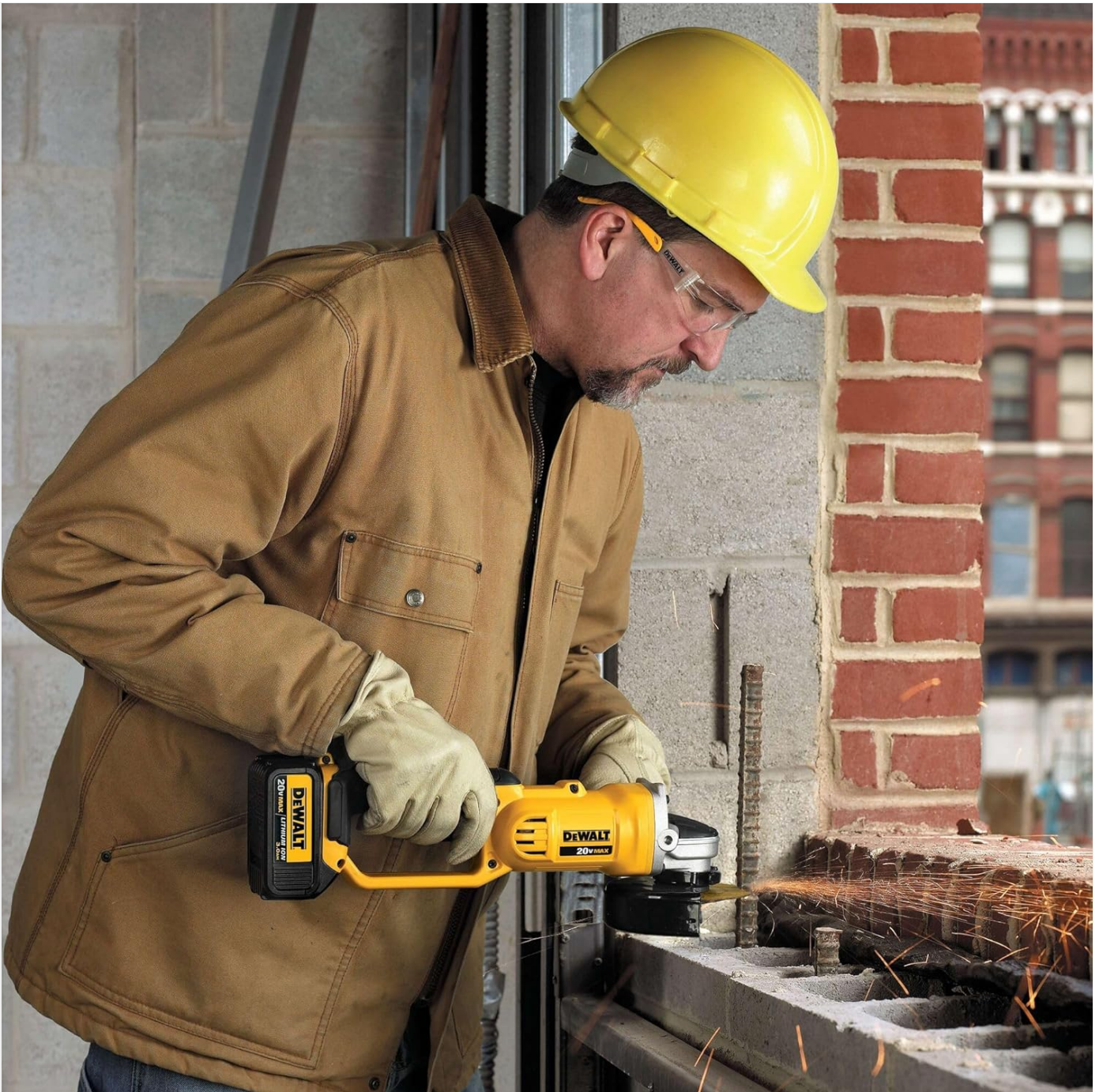
Figure 5.2: Rebar Cutting Application. This image captures a worker using the DEWALT angle grinder to cut through rebar, illustrating the tool's capability for heavy-duty cutting tasks and the visible sparks generated during operation, emphasizing the need for safety precautions.
