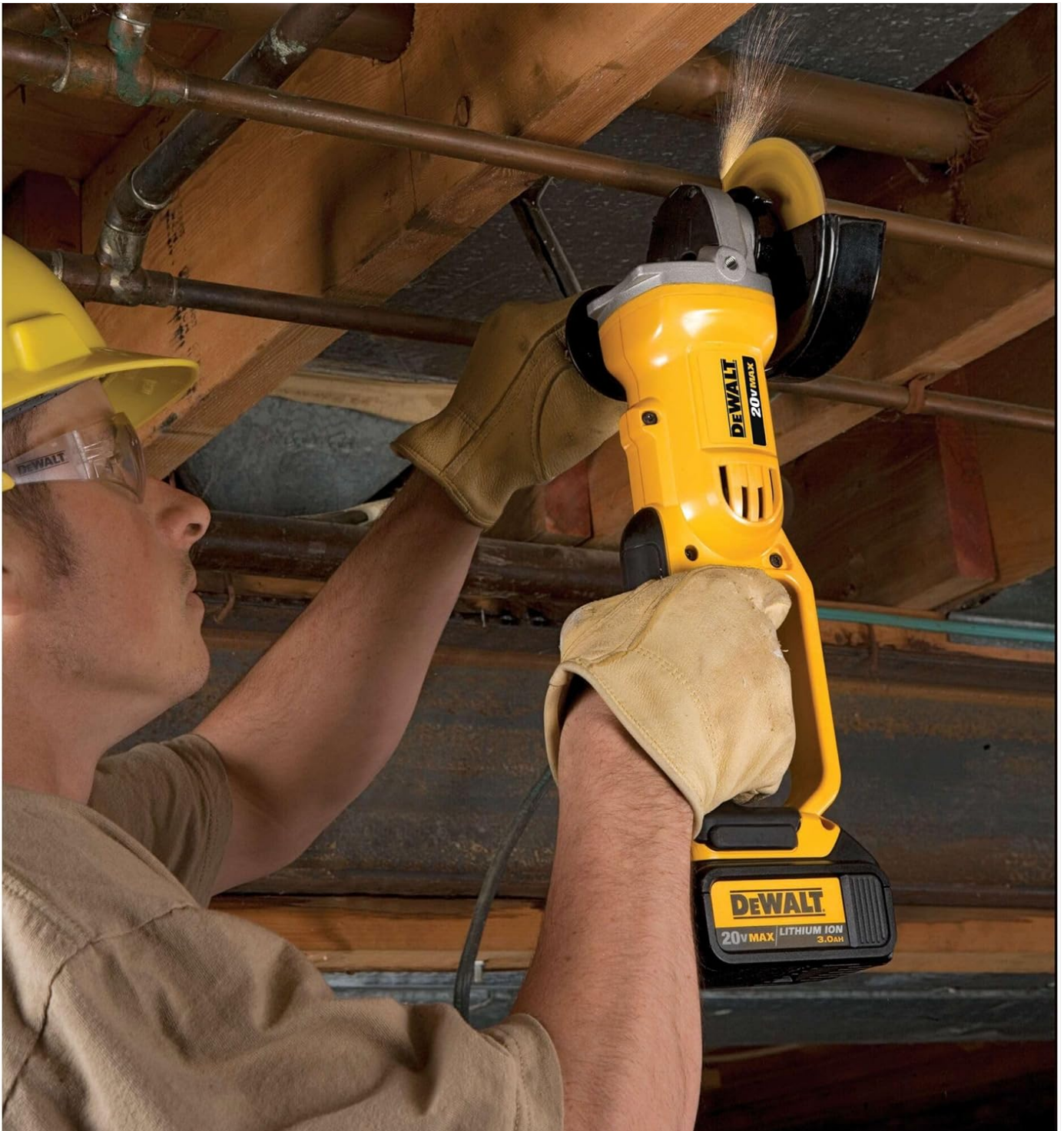
Figure 5.1: Overhead Cutting Application. This image shows a worker safely operating the DEWALT angle grinder to cut metal piping in an overhead position, demonstrating the tool's versatility and the importance of proper safety gear like glasses and gloves.
