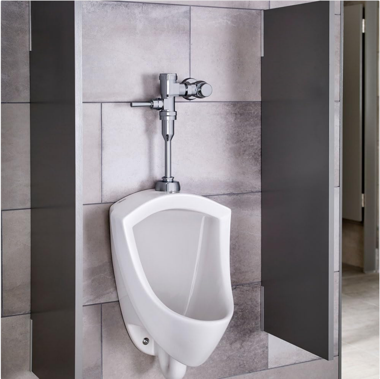
Figure 1: American Standard Ultima Manual Urinal Flush Valve installed on a urinal.
