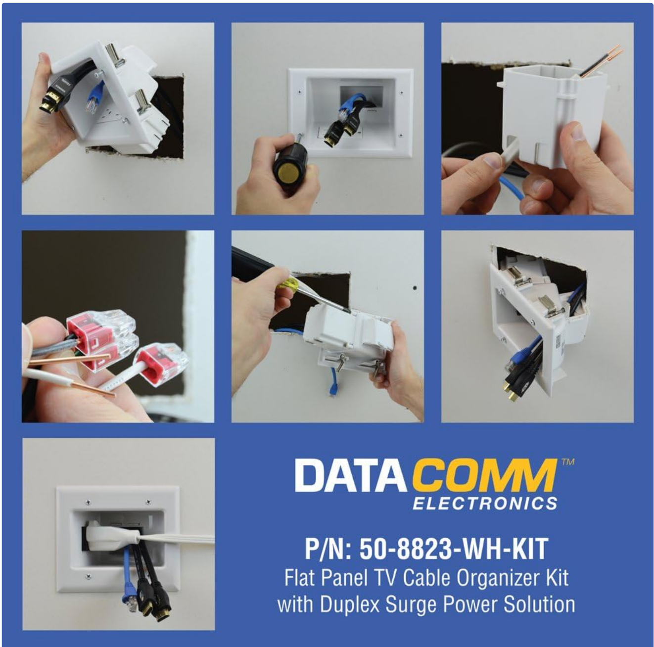
Figure 3.2: Visual guide demonstrating key installation steps, including cutting the wall, inserting units, and routing cables.
