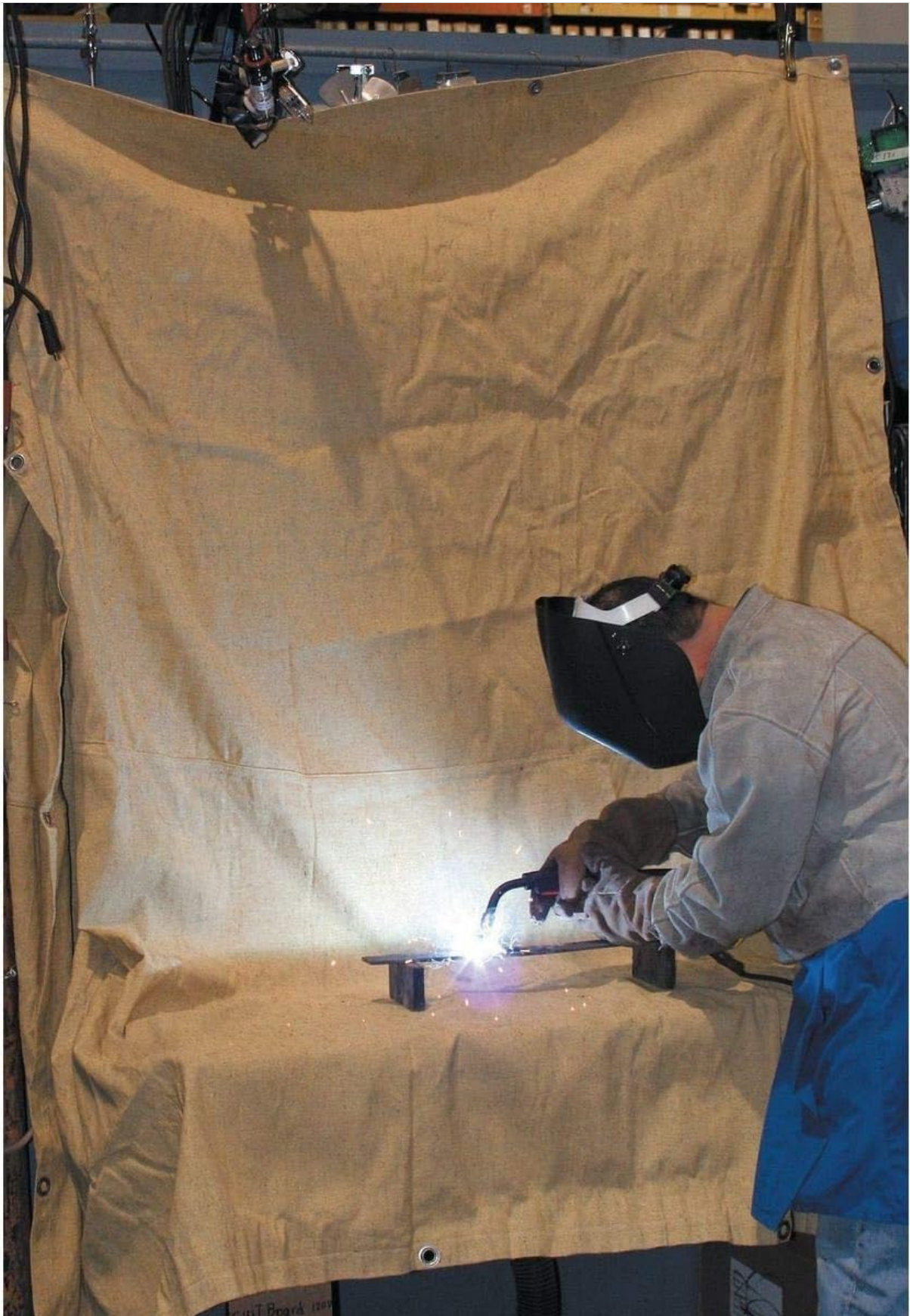
Figure 1: Proper use of the welding blanket to protect the surrounding environment from welding sparks and splatter. The blanket is positioned to create a barrier around the welding operation.
