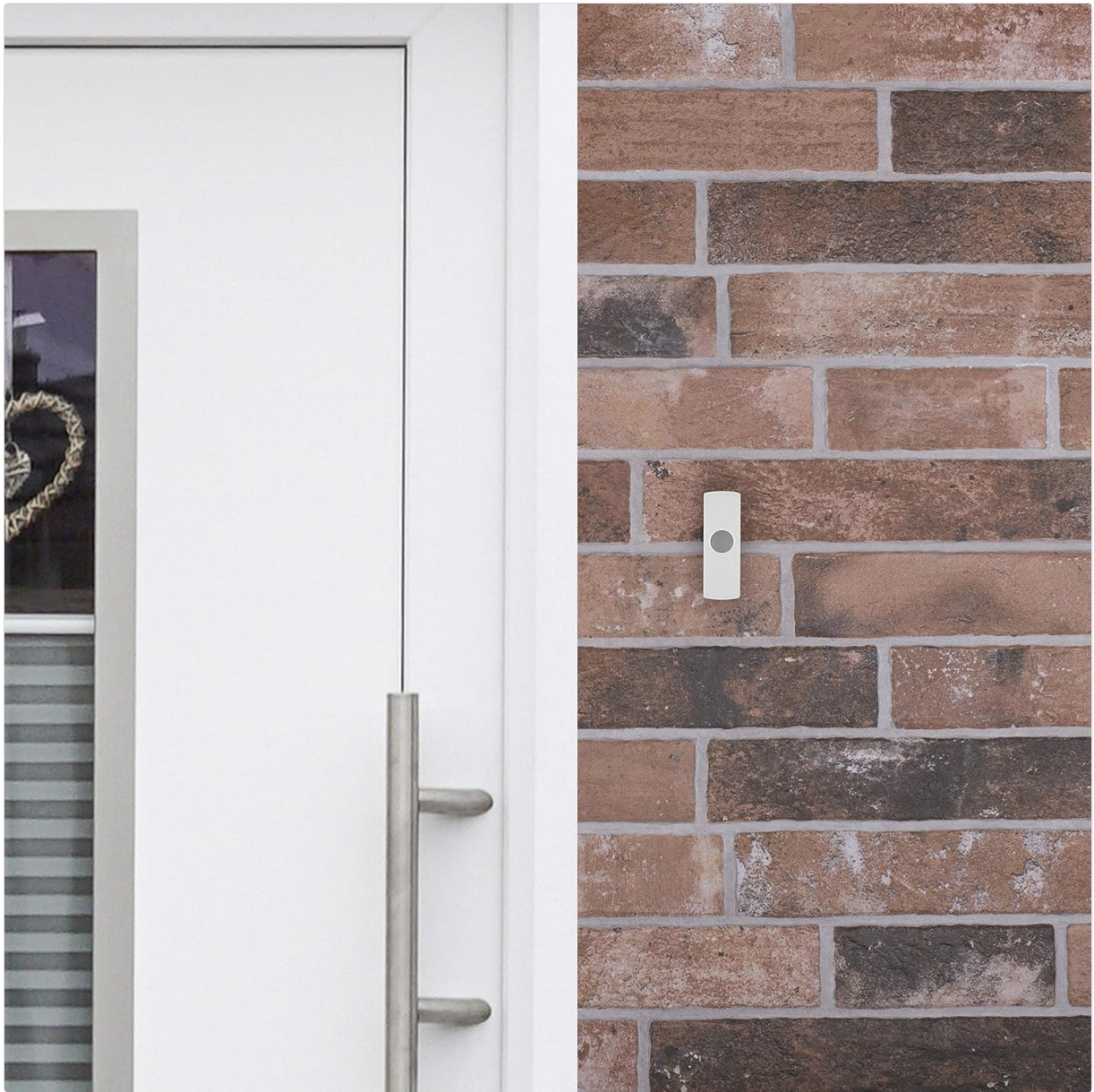
Image 3.2: The doorbell push button securely mounted on a brick wall next to a door, demonstrating a typical installation scenario.
