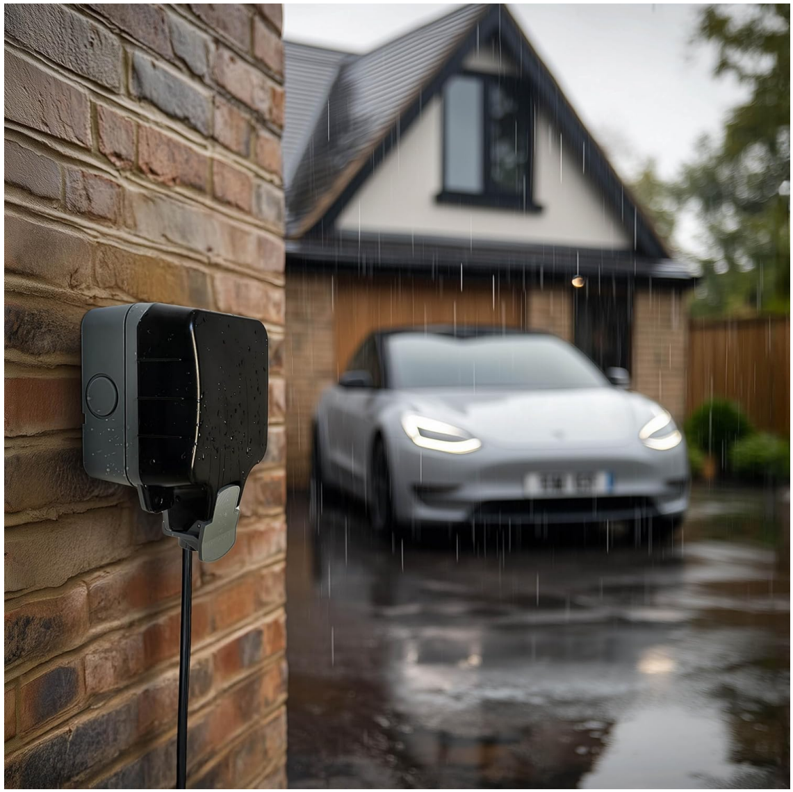
Image: The weatherproof socket installed on an exterior wall, providing power to an electric vehicle even in rainy conditions.
