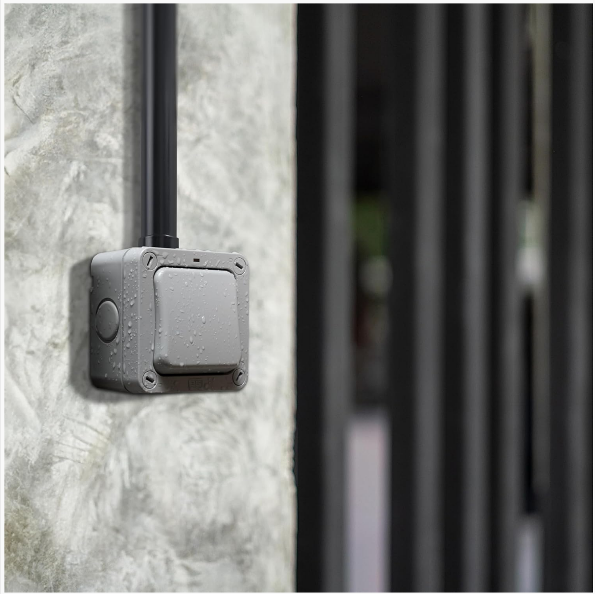
Figure 7: The BG Electrical WP12-01 switch installed on an exterior wall, ready for use.
