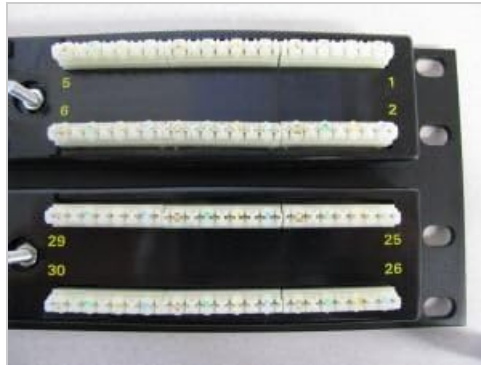
Figure 4.4: Detailed rear view of punchdown blocks, specifically for ports 25-30, showing color coding.
