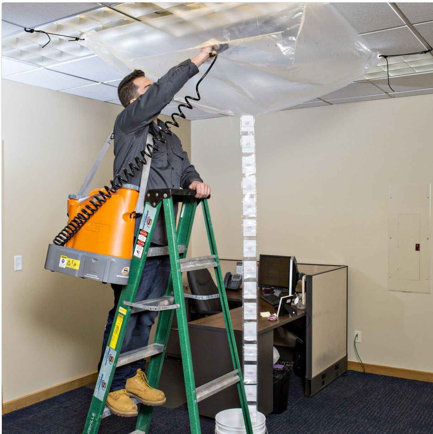
Image: A technician on a ladder cleans a ceiling-mounted HVAC unit. The CoilJet is used to spray the coil, with a collection bag (coil bib) positioned underneath to catch the cleaning solution and debris.
